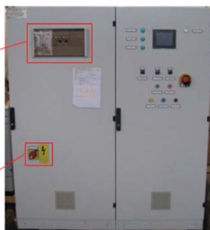
Fig.35 Electric Control Panel
