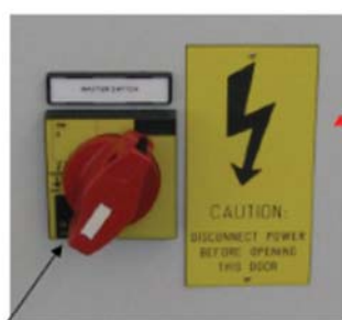
Fig.34 Main Power Switch
